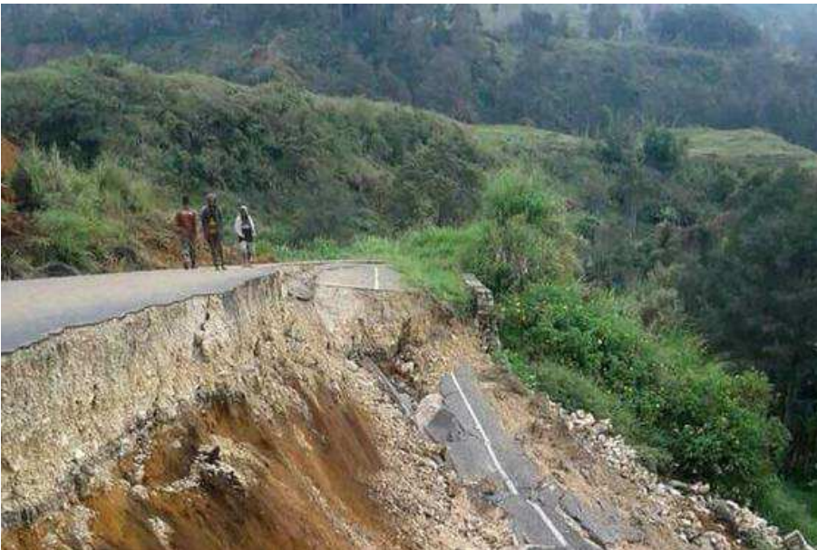
A road damaged by a February earthquake near Mendi in Papua New Guinea's highlands region. The earthquake killed more than 100 people. PHOTO: MELVIN LEVONGO/AFP/GETTY IMAGES
